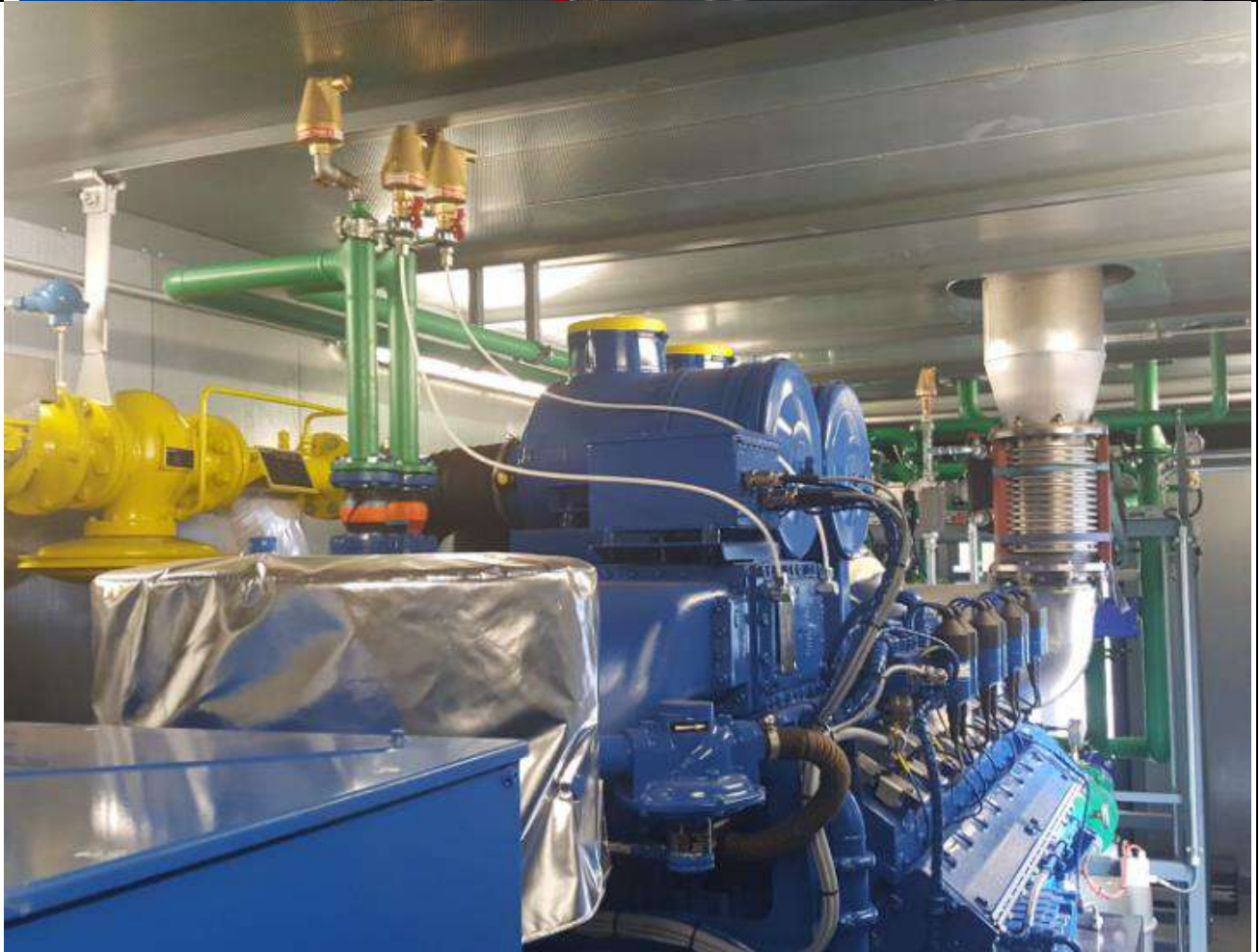
CIU CHP Plant for Biogas Project.
