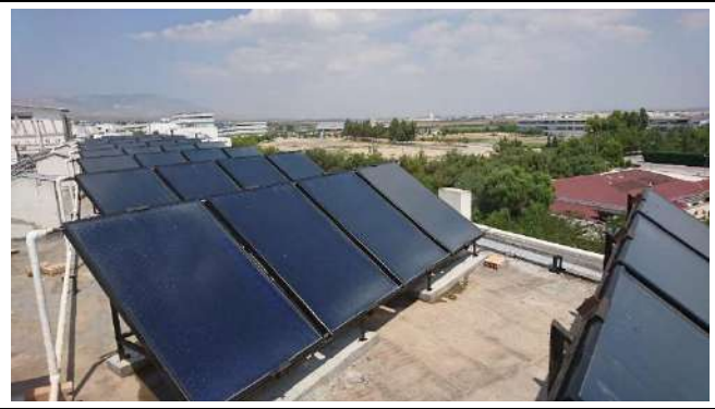
Solar Thermal Panels
